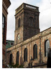
St Ann's Church, Manchester: Originally built in 1712 with Collyhurst sandstone, much of which has required repair or replacement.
